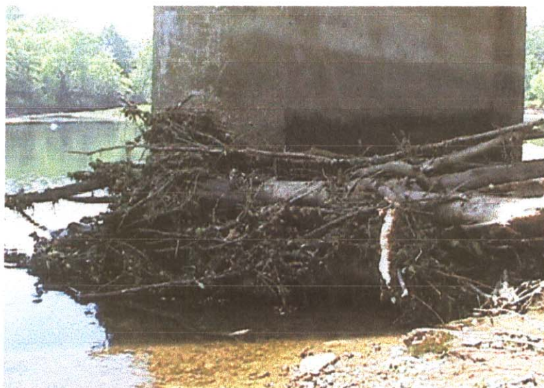
DRIFT AT PIER #2
